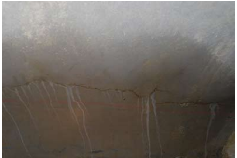
Fig. 3: A typical crack in the pipe wall
