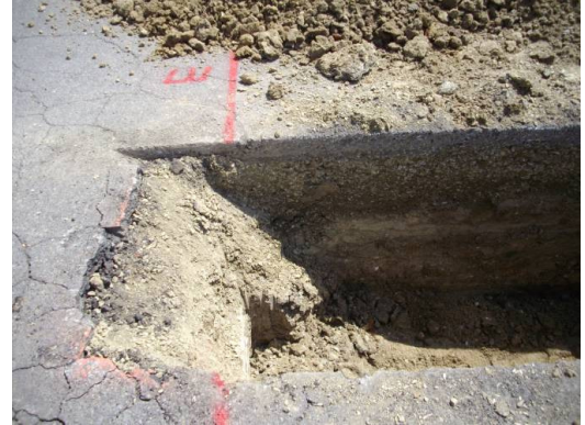
Figure 10. Electrical line crossing the air pipe.
