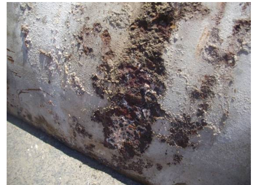
Figure 9. The host pipe was corroded.
