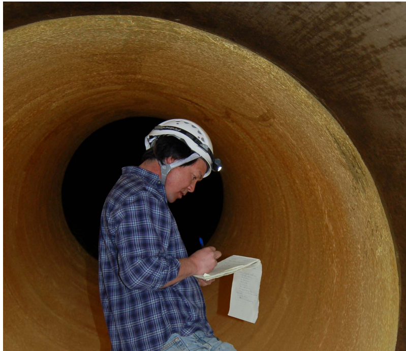
Figure 1. MWD inspector observing condition of the Tyfo Fibrwrap system after 8-year in service history
