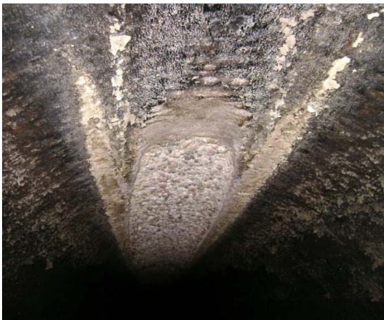
Figure 2. Surface Corrosion and exposed aggregates.
