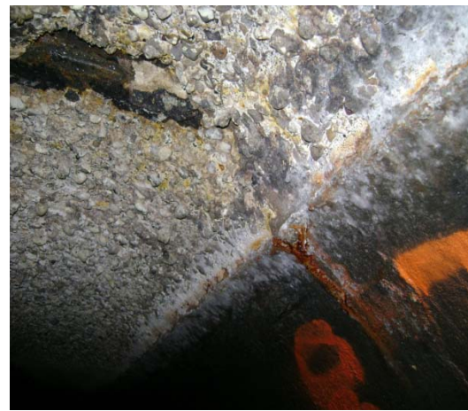
Figure 3. Spalling and exposed bell and spigot ring.
