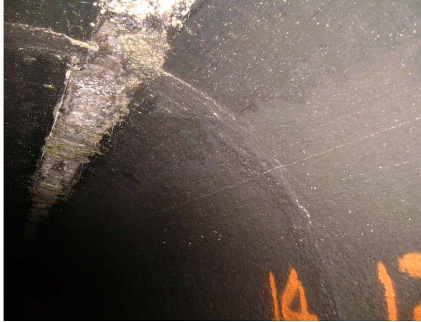
Figure 4. Early stages of corrosion at crown of pipe.
