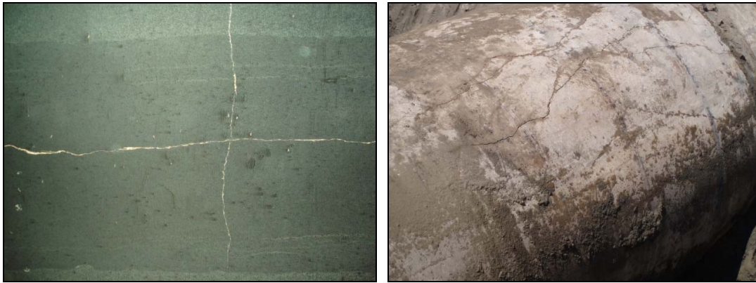
Figure 2 - Longitudinal cracks on pipe R329 (internal and external)
