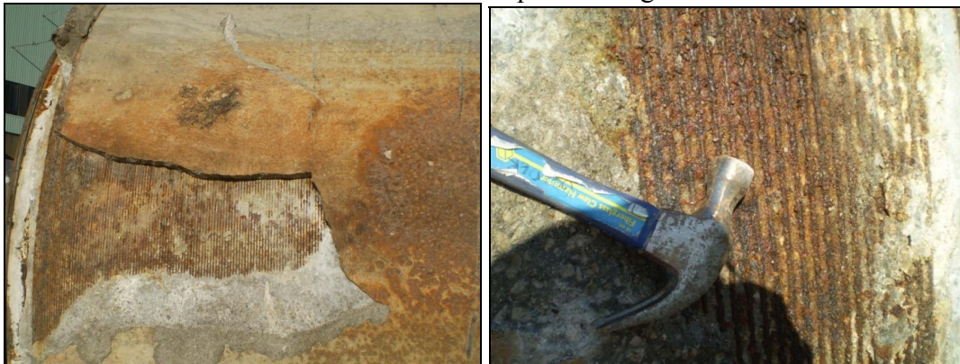
Figure 9 – Corrosion of Prestressing Wires
