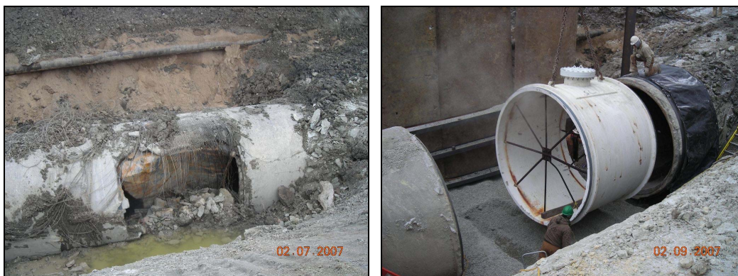
Figure 7 – Ruptured and repaired PCCP pipe
