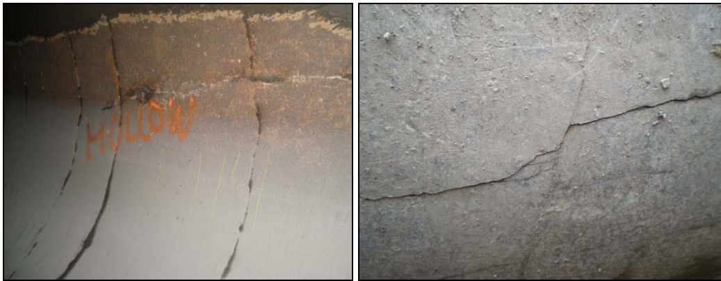
Figure 8 – Internal and External Longitudinal Cracks and Hollows
