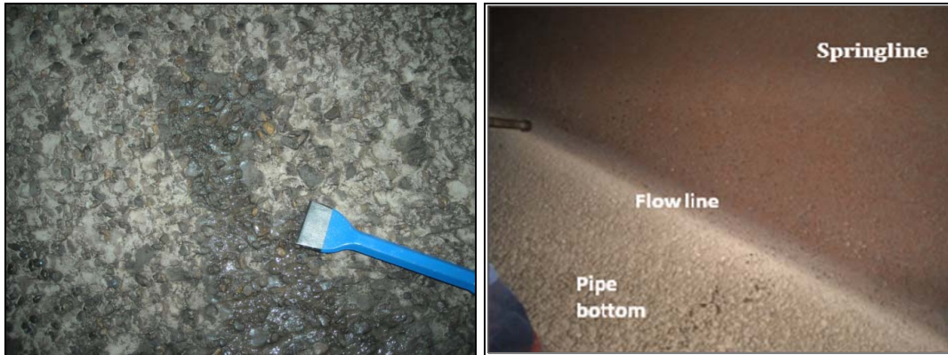
Figure 13 – Erosion at the bottom of the PCCP
