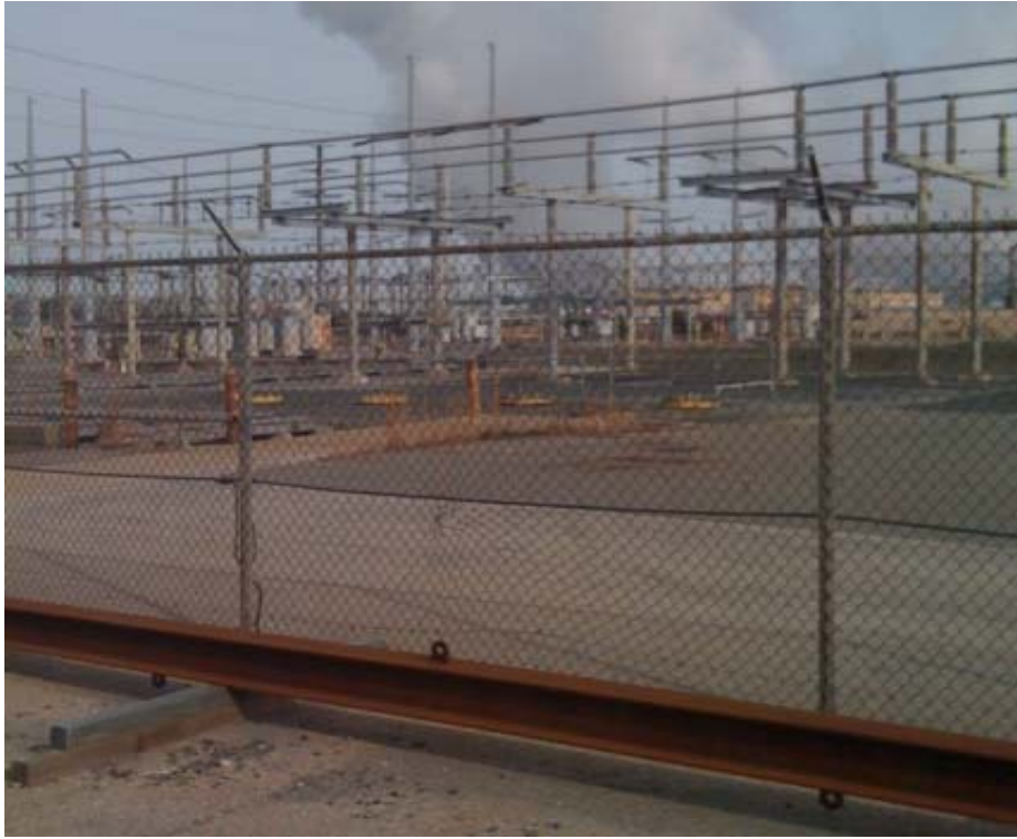
Figure 1. Power grid that lies on top of the PCCP line to be rehabilitated
