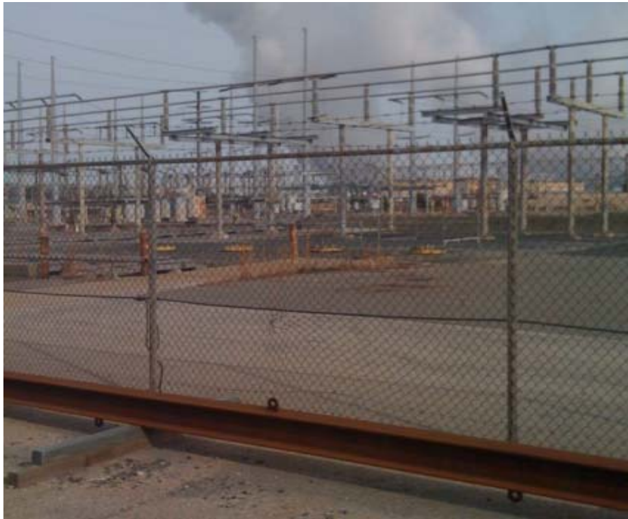
Figure 1. Power grid that lies on top of the PCCP line to be rehabilitated
