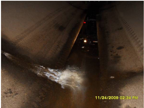
Figure 8 - Active Infiltration Defect
