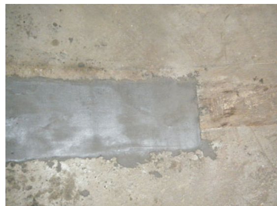
Figure 13 - Mortar repair and original mortar interface
