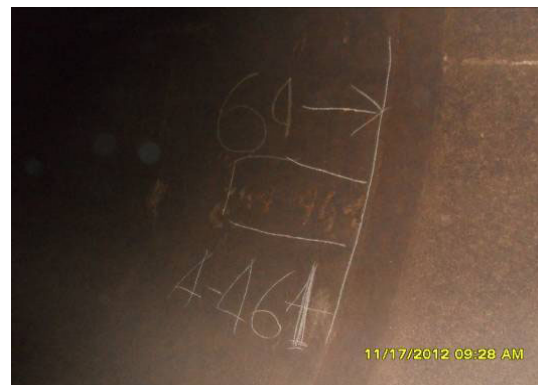
Figure 3 Internal pipe identification
