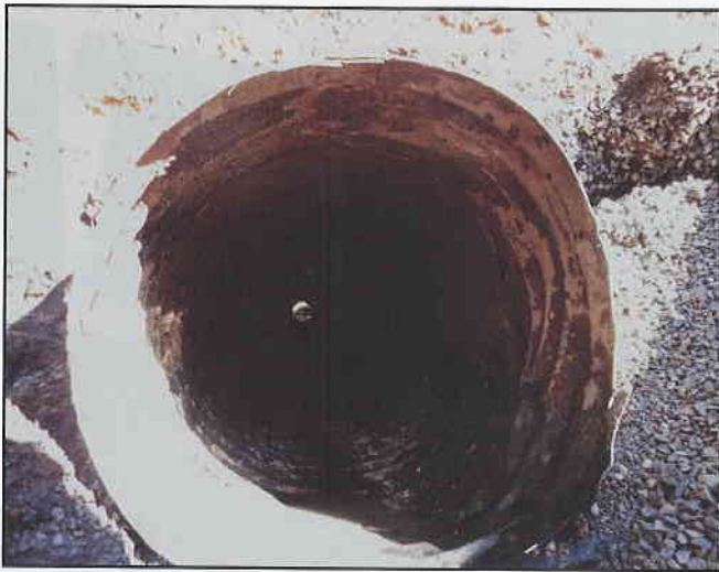
Figure 3. Highly corroded culvert at Arc Terminal
