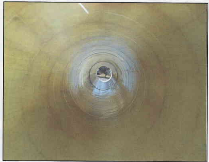
Figure 4. StifPipe at Arc Terminal – completed installation
