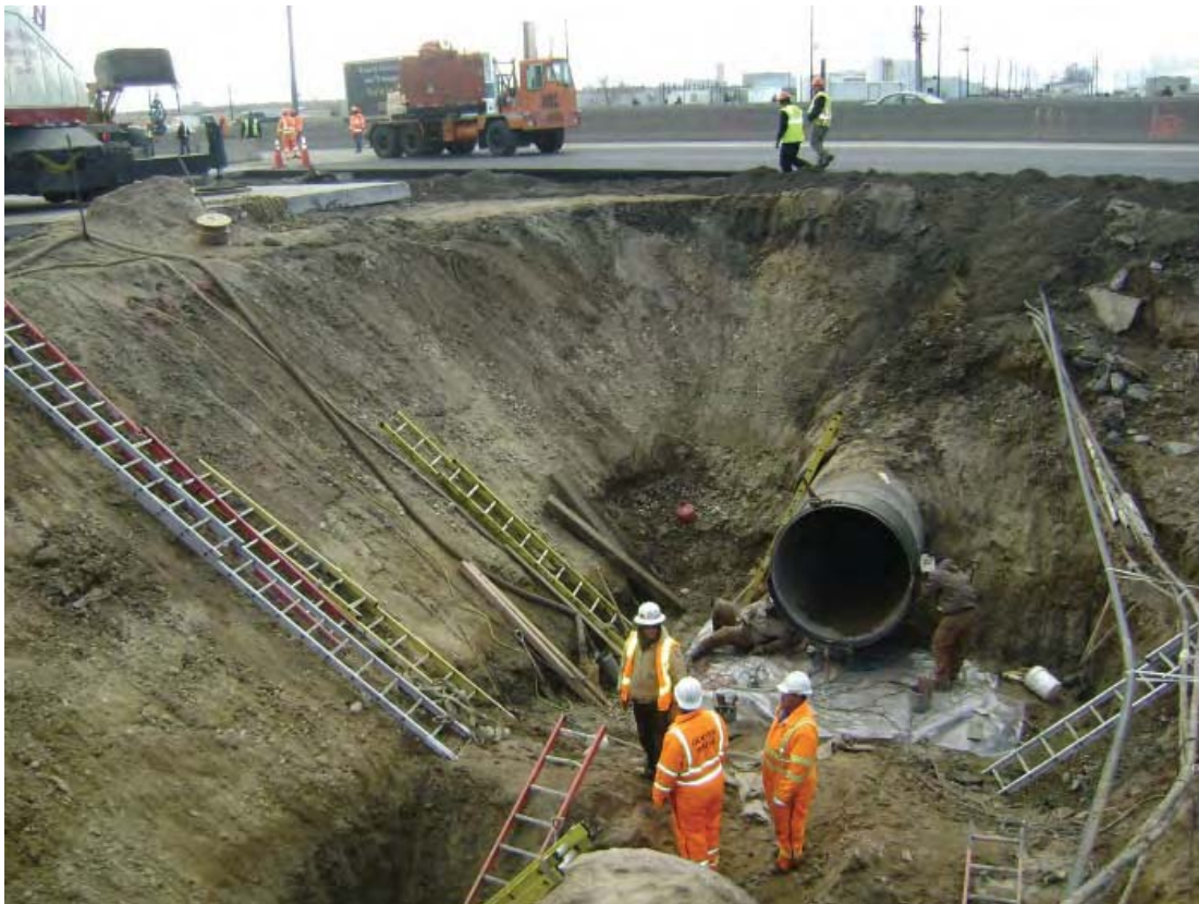
Figure 1. Failed pipeline segment for Denver Water (EPA 2009)
