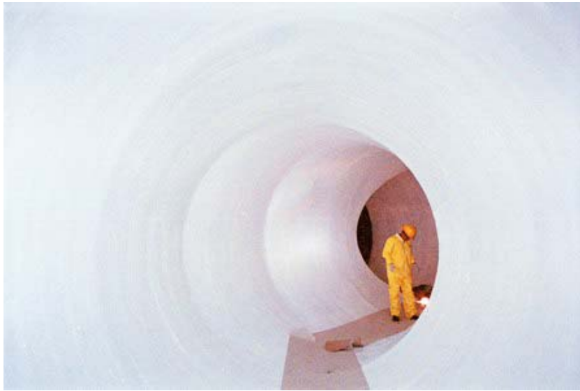
Figure 3. Interior View of Dominion Pipe
