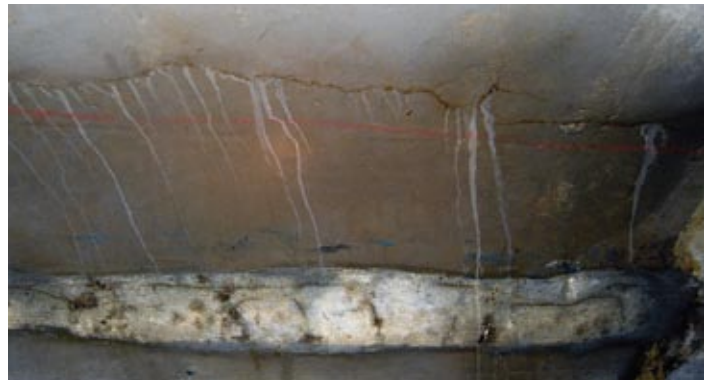
Fig. 3: Water seeping into pipeline
