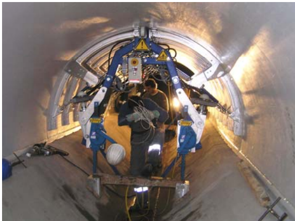
Figure 15. Erection device to press the 4 m long polyethylene sheets against the culvert
