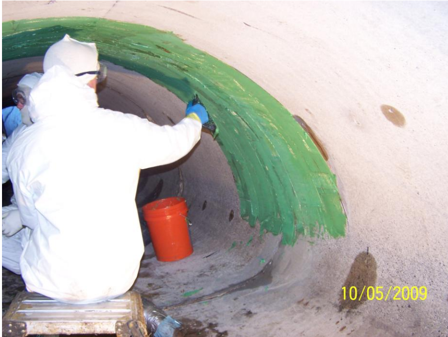
Photo 143: QuakeBond™ J201TC Tack Coat being installed. Does not need to be placed on the bottom.
