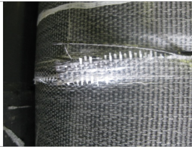
Fig. 12. Close up view of failure region
