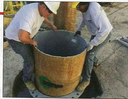
↑ Figure 2. A prefabricated FRP system (Stifpipe) being inserted into a vertical access hole.
