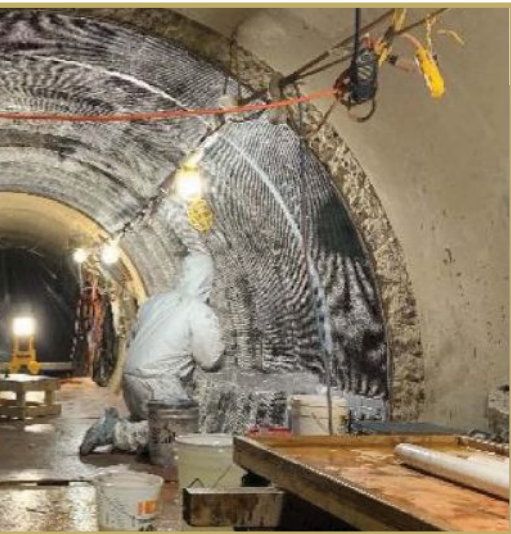
Figure 2. Installation of a carbon fiber layer of StifPipe by FRP Construction crew.
