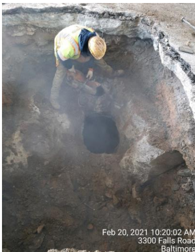
Blow hole on the pipe
